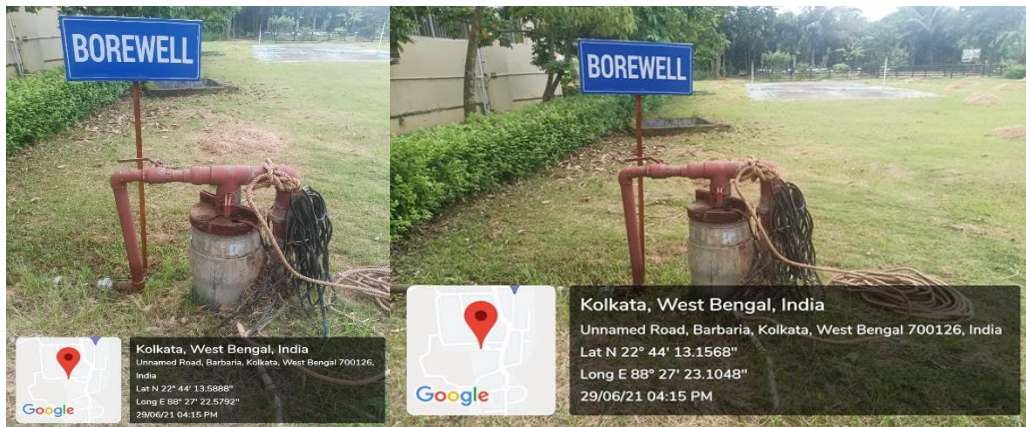
Fig 1: Installed Borewell within the campus
