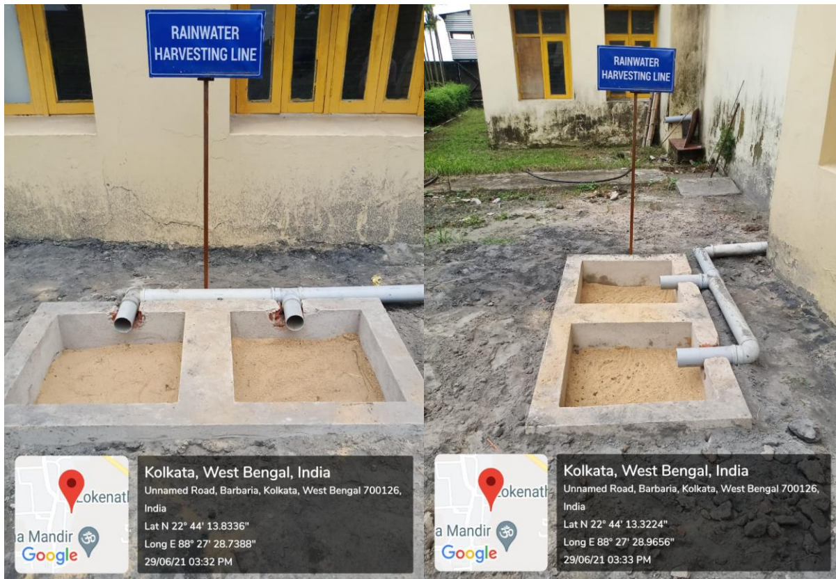
Fig 1: Rainwater harvesting infrastructure within the University campus
